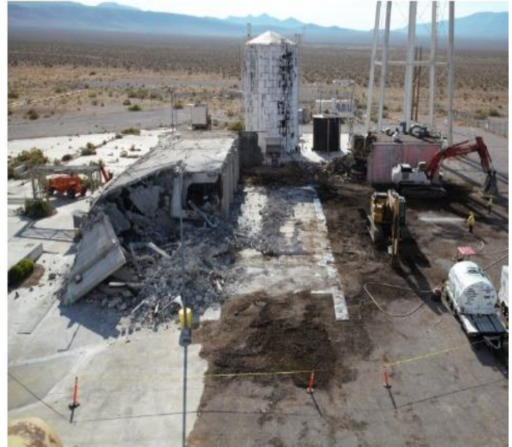
An overhead view of Test Cell C Facility on the second day of Building 3220 demolition.
