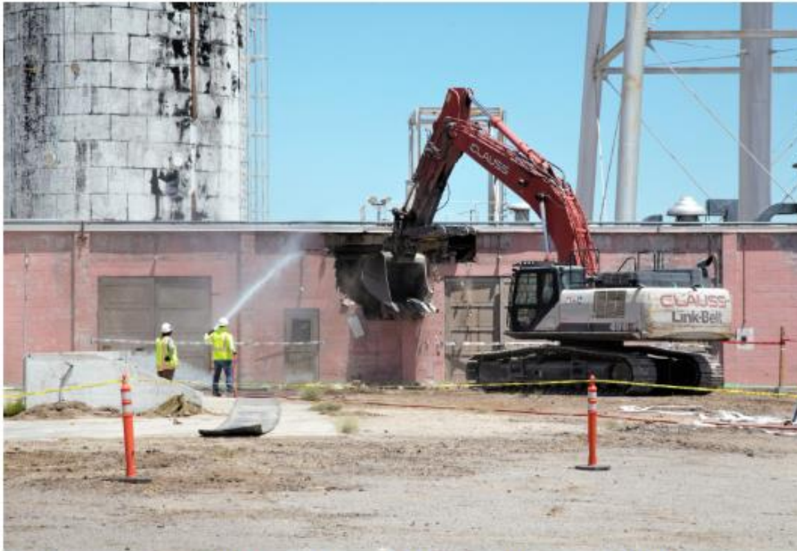
EM crews begin demolition of Building 3220 at Test Cell C at the Nevada National Security Sites in late June.
