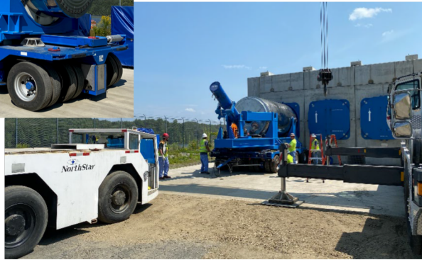
Transfer into the HTS (Storage Vault)
