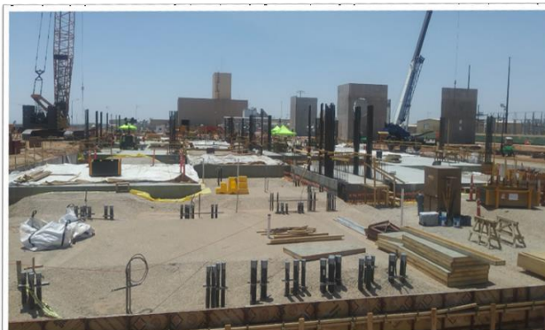
New Filter Building construction as part of the SSCVS, which will increase HEPA filtered air to the WIPP underground, enhancing worker safety throughout the mine.
