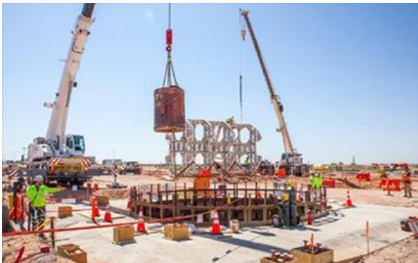
A bucket of excavated dirt is lifted out of the utility shaft.
