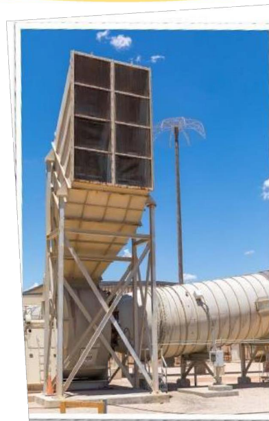
Restarting 700 fan provides increased air flow to workers.
